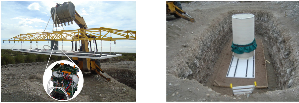
Figure 8. ( lhs ) First module buried at the Observatory site, the insert shows the electronics inside its enclosure; ( rhs ) Muon counter placed over sand bed with service pipe installed, about to be buried.
